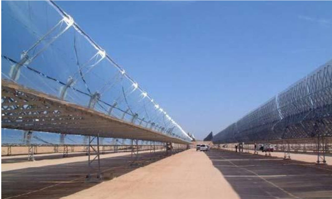
Figure 10: Parabolic mirrors of the solar thermal power plant, Cyprus
