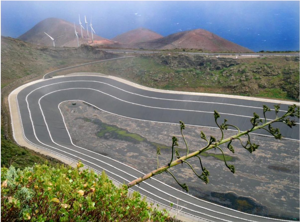
Figure 8: Construction of the upper reservoir of the hydro storage plant, El Hierro (Canary Islands)
